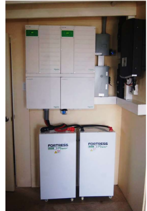
13.6 kW/30 kWh ESS
