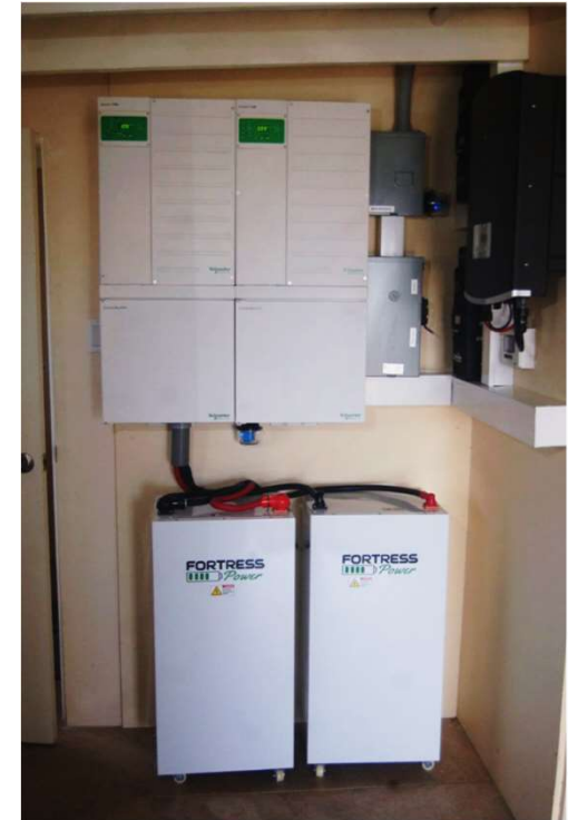
13.6 kW/30 kWh ESS
