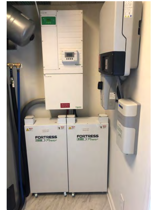
6.8 kW/30 kWh ESS
