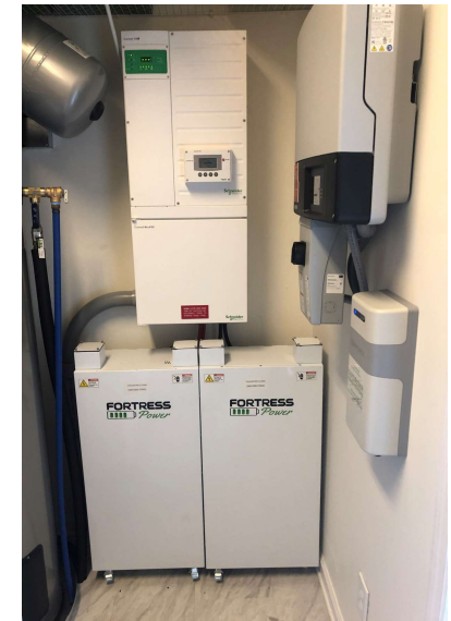
6.8 kW/30 kWh ESS
